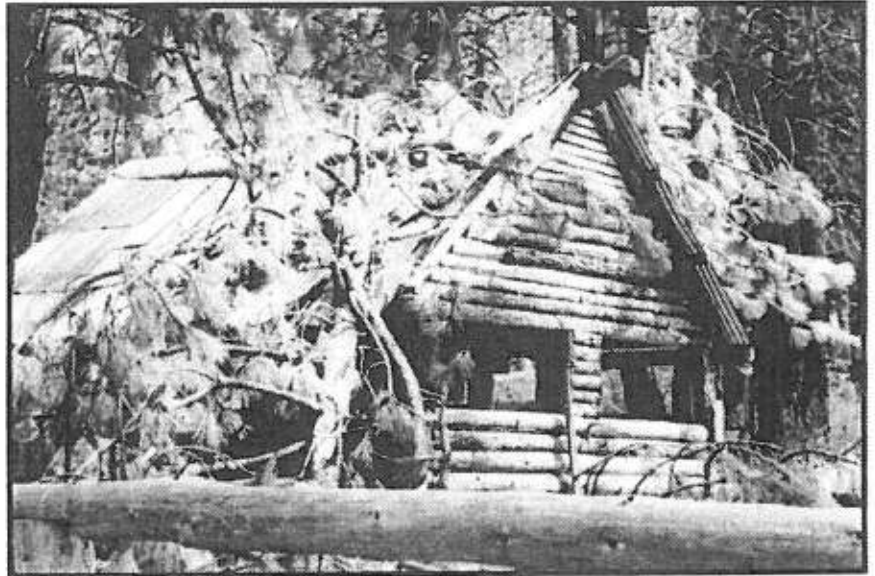
Cooking and Dining Cabin received major damage from a fallen tree.
