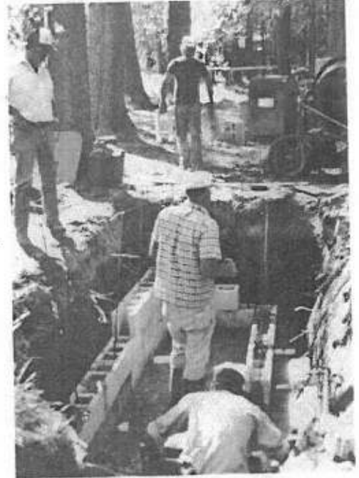
Dennis hauls blocks for O.B. and Dutch to set in place as Tommy observes. Note water in bottom of hole built to drain!
